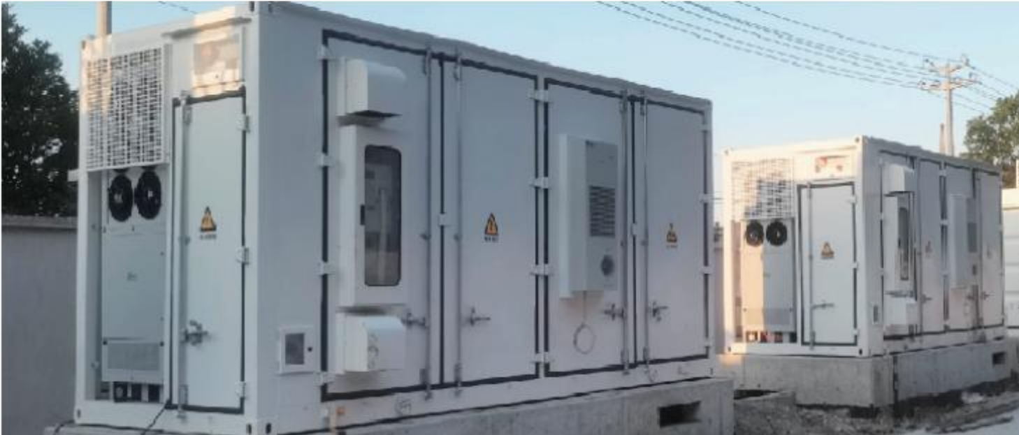
The 6.88 MW / 13.76 MWh energy storage system is located in Nanjing, China
