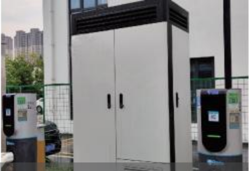
The 500KWh energy storage system is located in China's Anhui Province.
