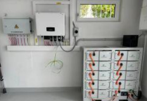
C&L 20KW / 45KWh The energy storage system is located in Nigeria.
