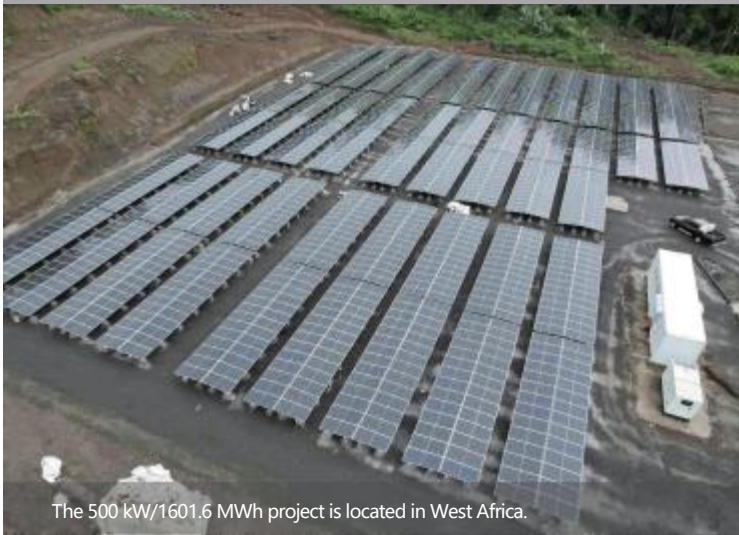
The 500 kW/1601.6 MWh project is located in West Africa.
