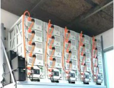
C&L 100KW / 300KWh The energy storage system is located in Nigeria.
