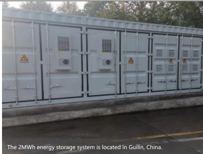
The 2MWh energy storage system is located in Guilin, China.
